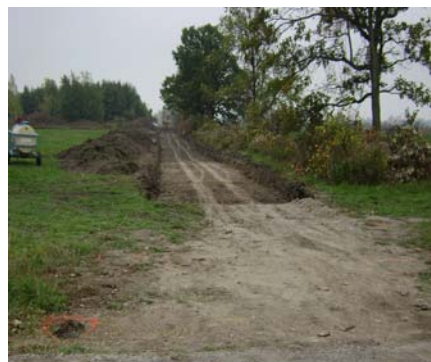
Photo (left) of first road being prepared at the Mohawk Point Wind Farm. Roads will be roughly 5m wide during construction prior to being returned to 4m permanent road width.
