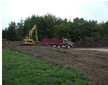
Photo (left) of preparation of roads in advance of the digging of foundation pits. Each foundation will be comprised of 37-40 truck loads of cement and 27 tons of rebar.
