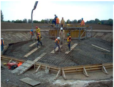
The photo to the left shows the rebar and form being prepared for the turbine foundation. Each turbine foundation is comprised of roughly 327m3 of concrete and 27,000 pounds of rebar.
