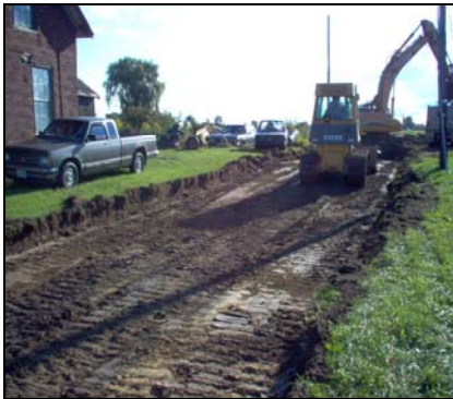
Photo of one of the access roads under construction as part of the Frogmore Wind Farm, near Port Burwell, Ontario. The Frogmore and Cultus Wind Farms are expected to meet the electricity requirements of over 3600 Ontario households.
