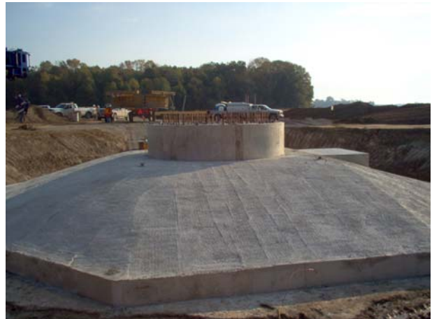
Photo of completed foundation prior to back filling the excavation pit. Notice the 120, 10 foot long anchor bolts used to attach the base of the turbine to the foundation. Each bolt has a diameter of 1 & 3/4 inches.
